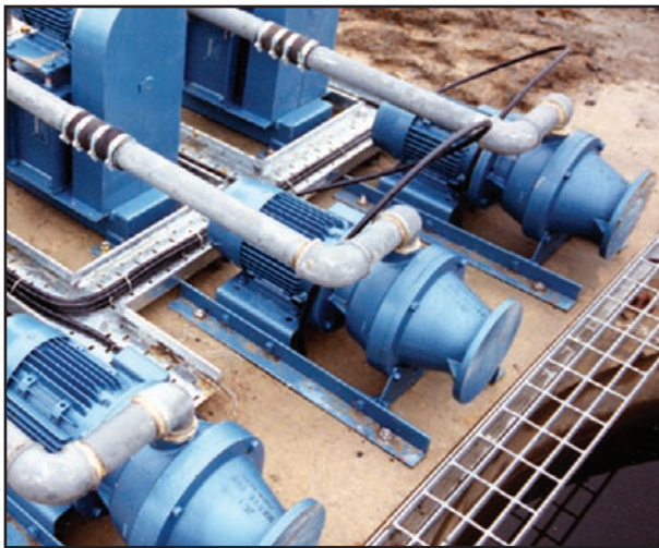
M18 Macerators, part of a Mutrator system installed to macerate settled sludge and storm tank effluent.
