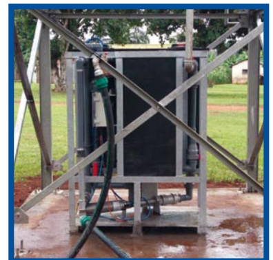
Mono Solar Filtration Unit designed in conjunction with GE.
