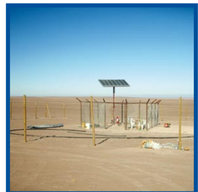
Mono Solar Sun-Sub System installed.
