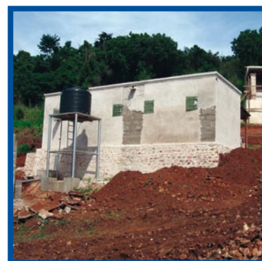
The new water supply at the Sesemi Museum.
