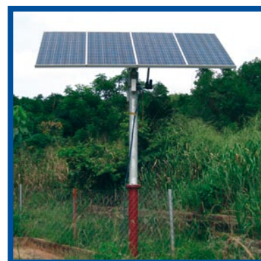
The 600W Tracking Array is mounted on a long pole to keep it out of reach.
