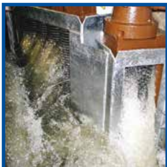
Discreen and Muncher screening and macerating waste water
