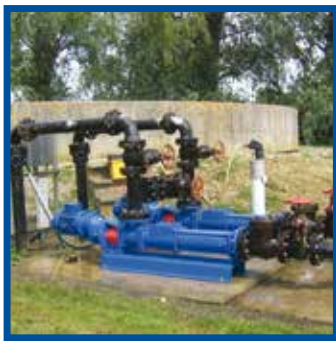
Transfer pumps at a WWTW's pumping sludge
