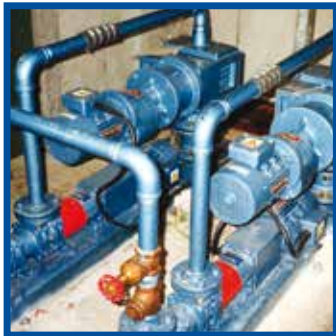
Packaged pumping system transferring raw sewage
